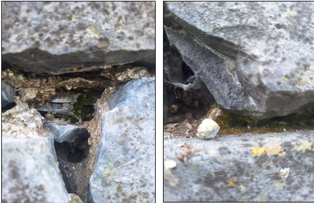
Plate 19 Mortar was noted as competent and strong; while pointing is missing, the bedding mortar is solid.
