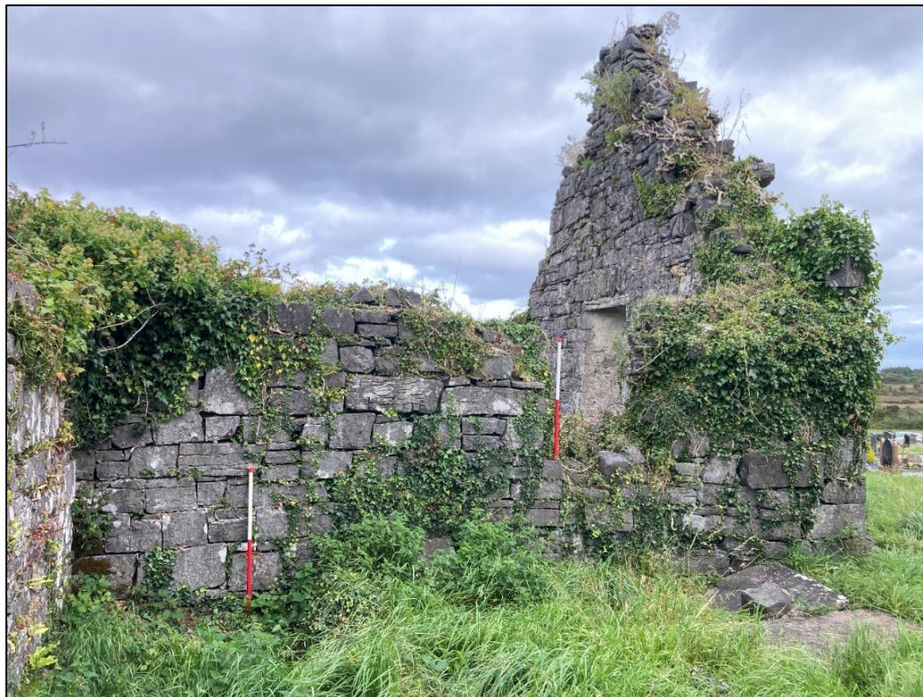
Plate 14 South elevation showing fallen masonry
