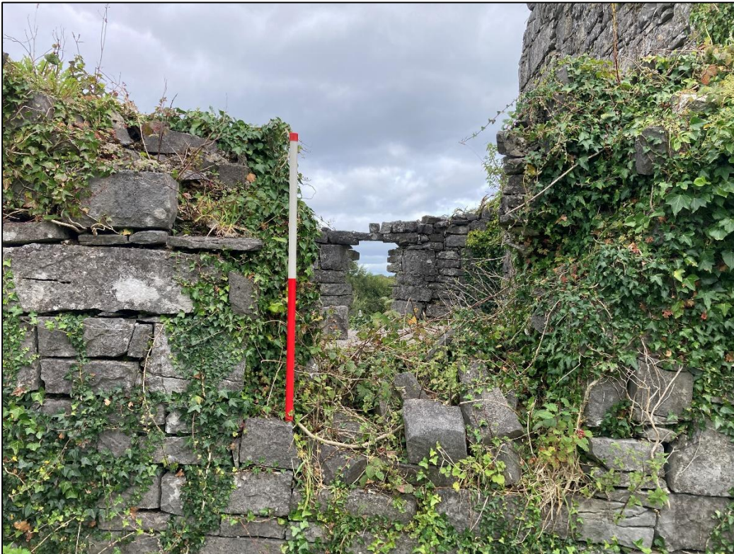
Plate 16 South elevation of the nave, east end. Window opening where window masonry has been lost.
