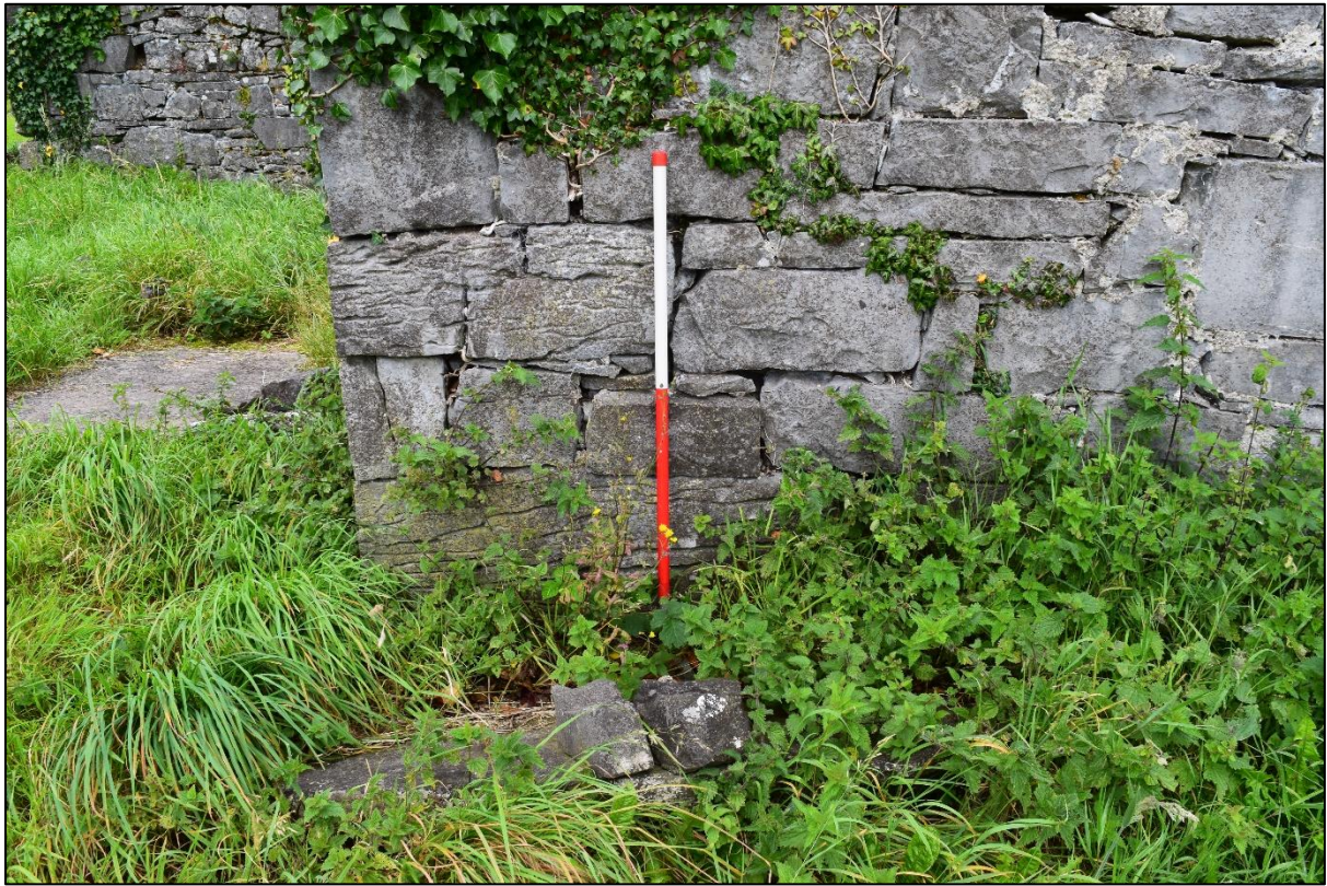
Plate 21 East elevation exterior: fallen masonry, carved coping stones may be part of the architectural fragments on the ground
