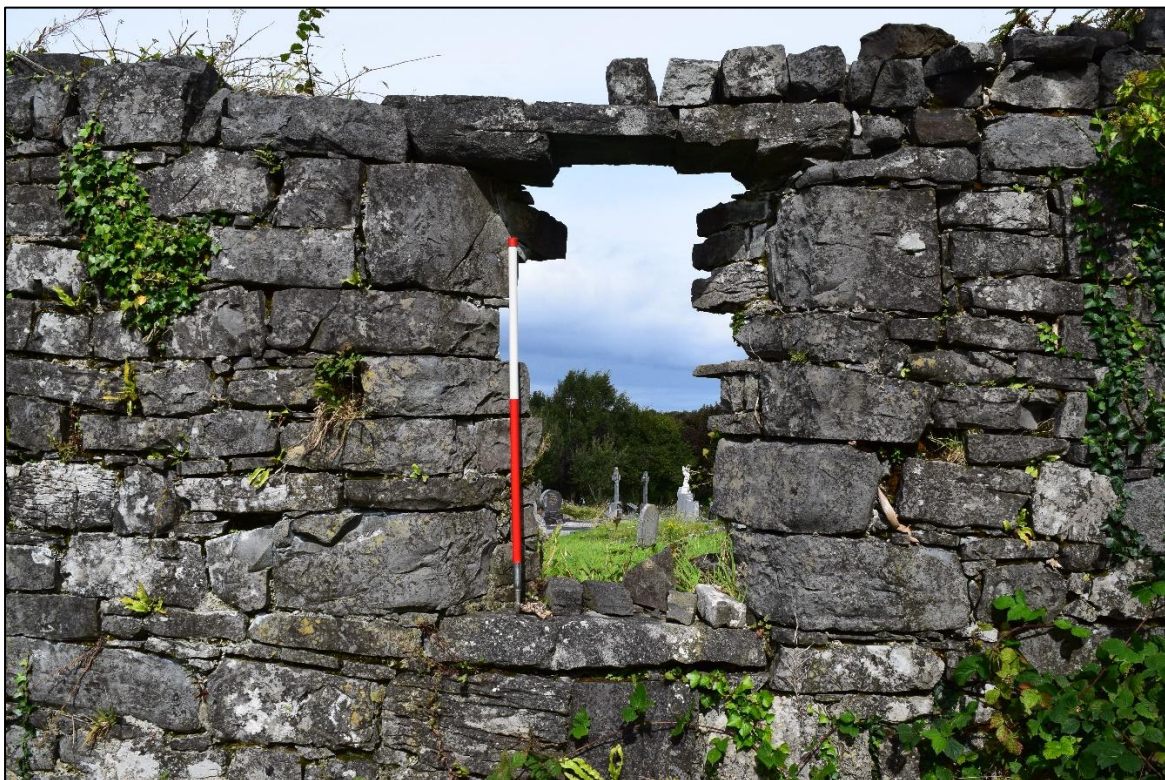
Plate 32: North elevation, interior view of missing window.
