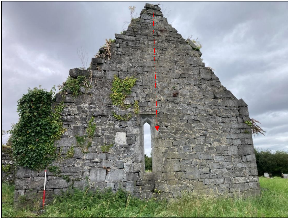
Plate 17 View of the east elevation; note the off-centre single ogee-headed light which is centrally located when viewed from the interior. Ivy has been previously treated and is affecting wall tops and requires removal, treatment with eco plugs and pointing and grouting in phase 1
