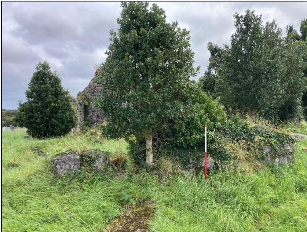
Plate 35: West elevation: The doorway which could help date the structure more accurately is gone, however, architectural fragments may still exist on the ground.
