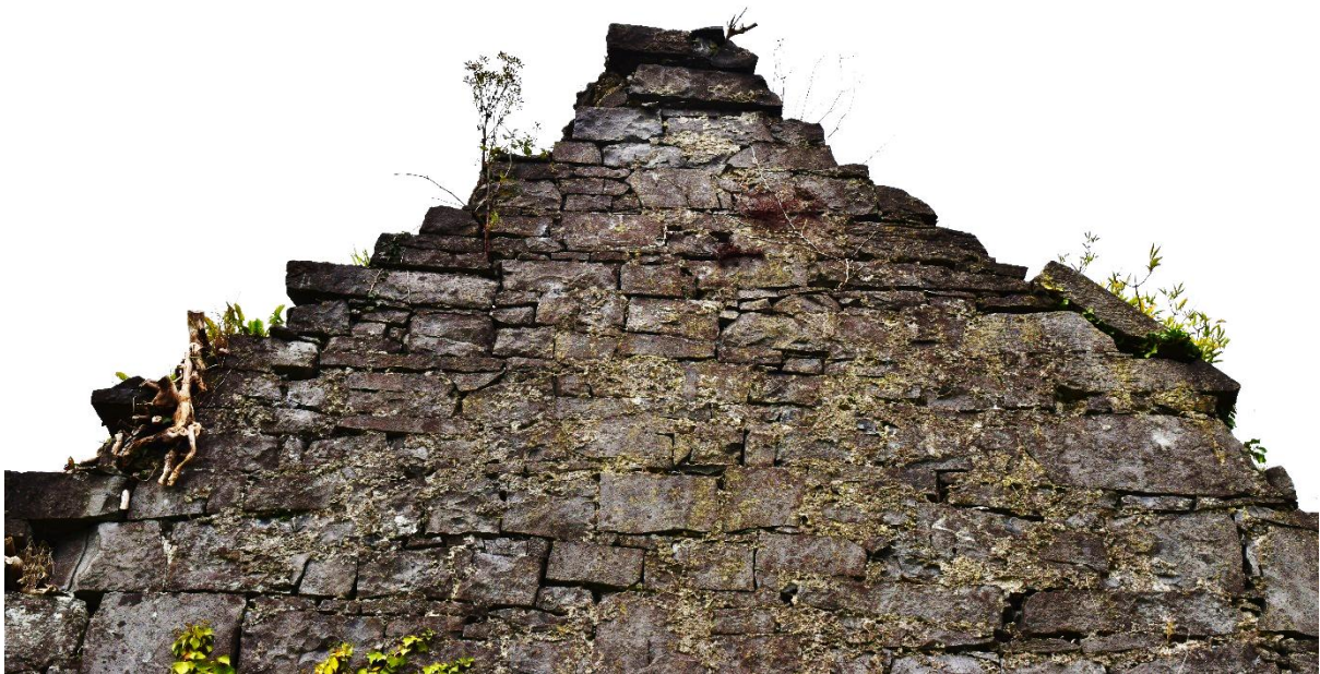
Plate 20 View of the East Gable (exterior): coping has been lost with only two pieces remaining.
