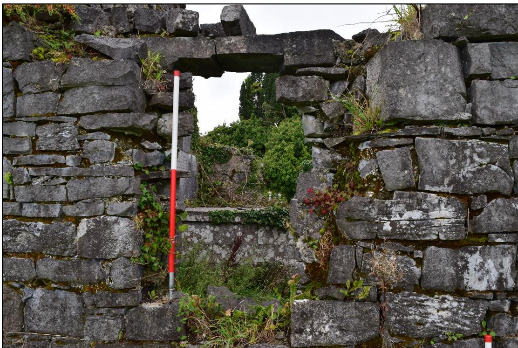
Plate 30: North elevation, window surround has been lost. Cracked lintel requires conservative repair as per Sketch B (Appendix 4)
