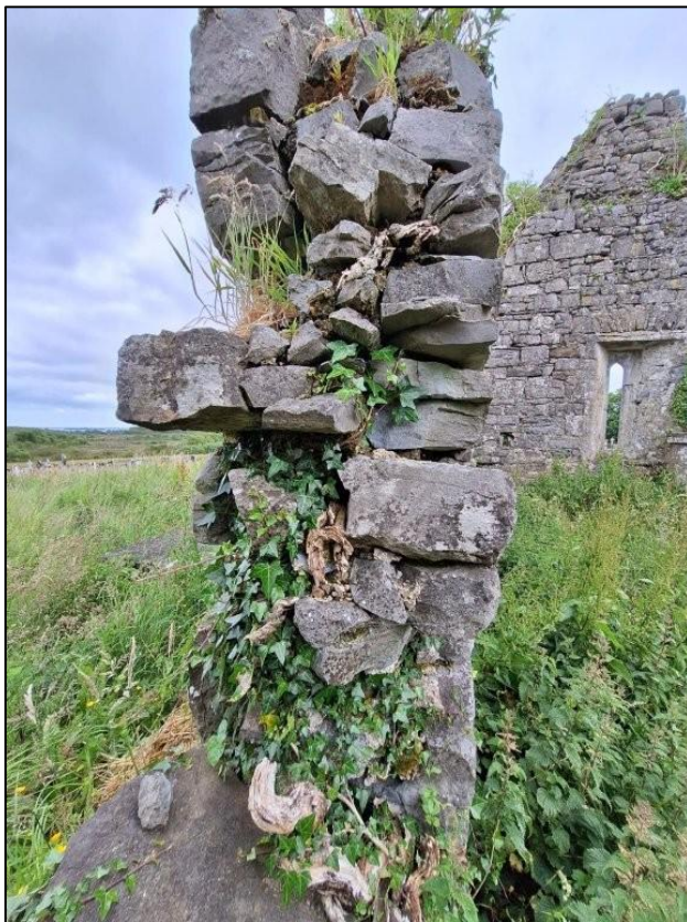
Plate 34: Typical wall construction with fragile tops and edges requiring consolidation
