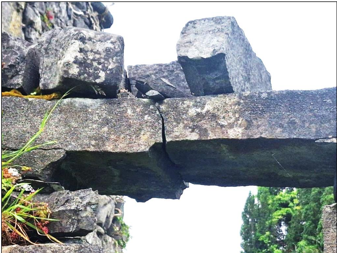
Plate 31: Detail of crack in lintel.
