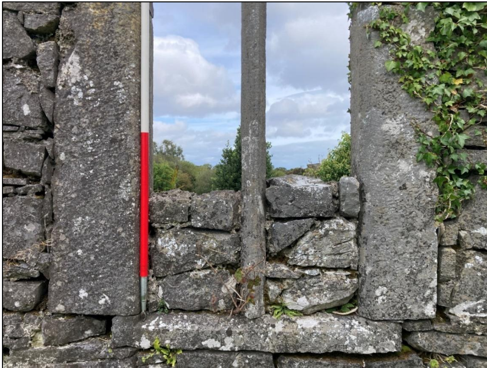
Plate 9 South elevation window partially blocked
